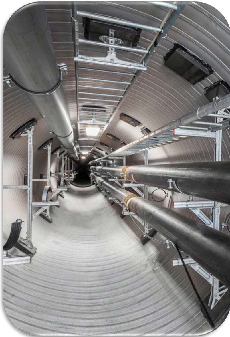
The Weholite 'infra tunnel' in a new city district in Linköping, Sweden collects pipes and cables in one easy-to-maintain tunnel
