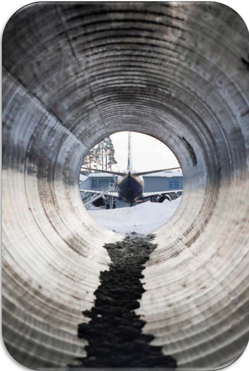
Soil drainage system at Nyköping airport, Sweden
